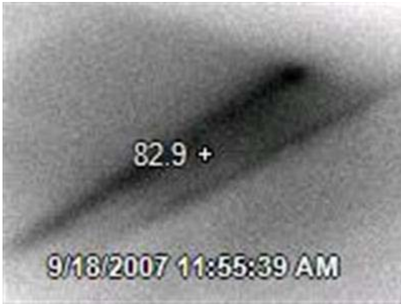
1.4 Picture 3 Black indicates moisture
