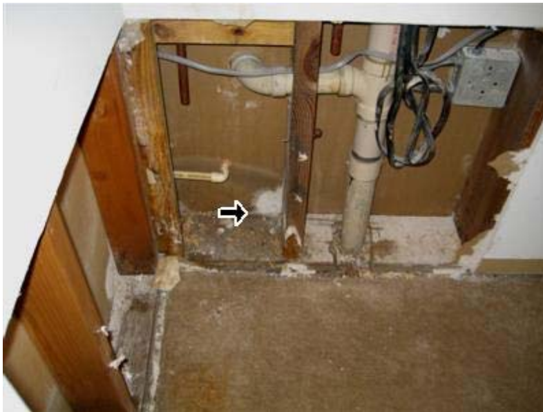
1.2 Picture 7 Master bedroom rear and side wall
